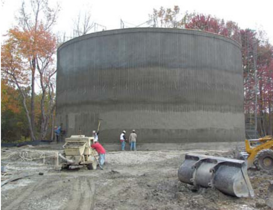
Fig 1. Sealit Multipurpose being applied to the outside of a large water tank.
